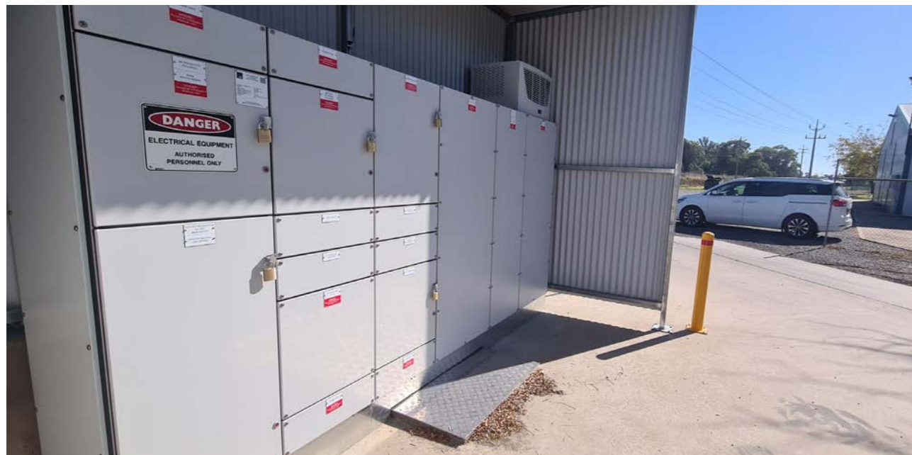
ClearScada System upgrade
