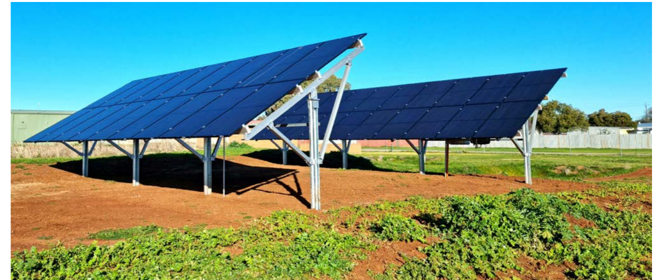
Whitton solar installation at Whitton Sewer Pump
