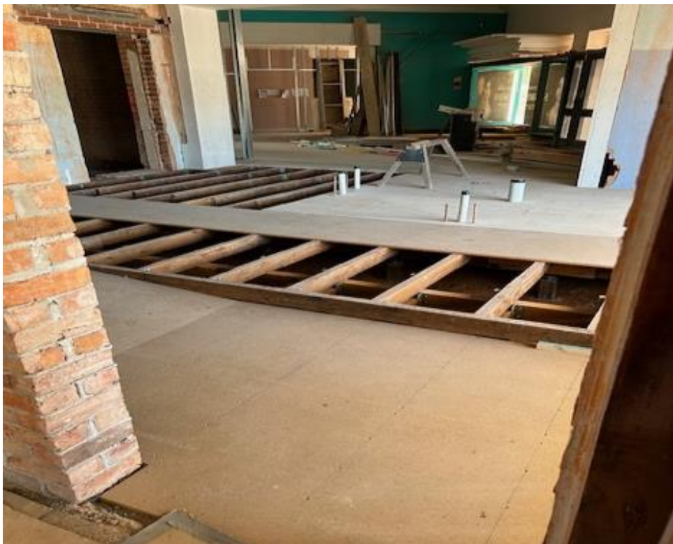
Figure 2 Cafe /bar flooring(recycled)
