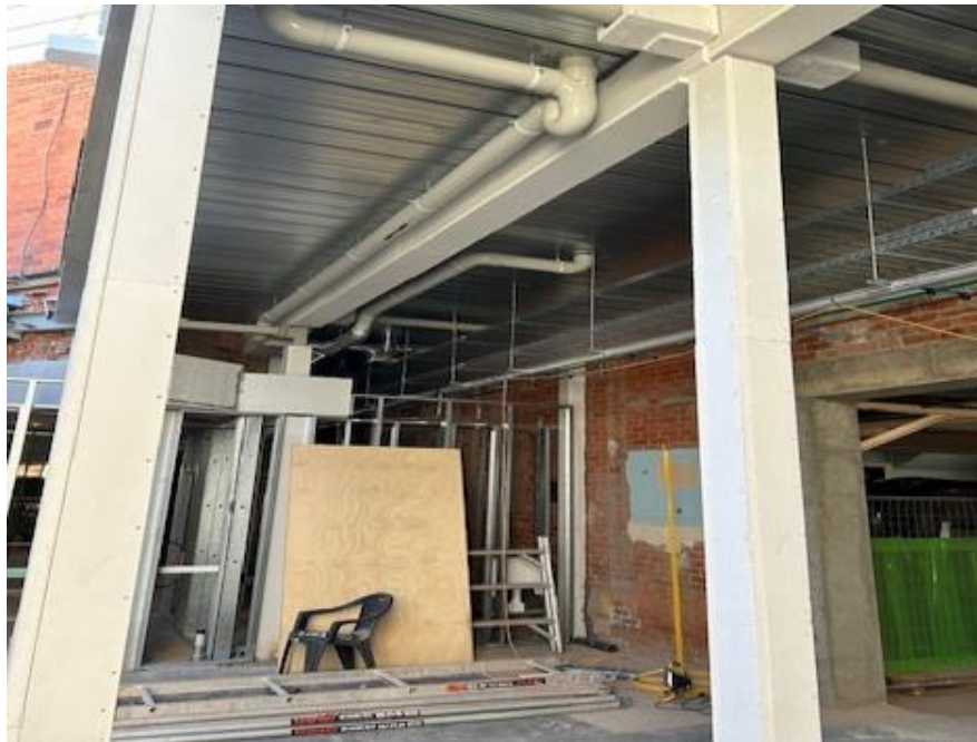
Figure 4 Electrical cable trays and drainage
