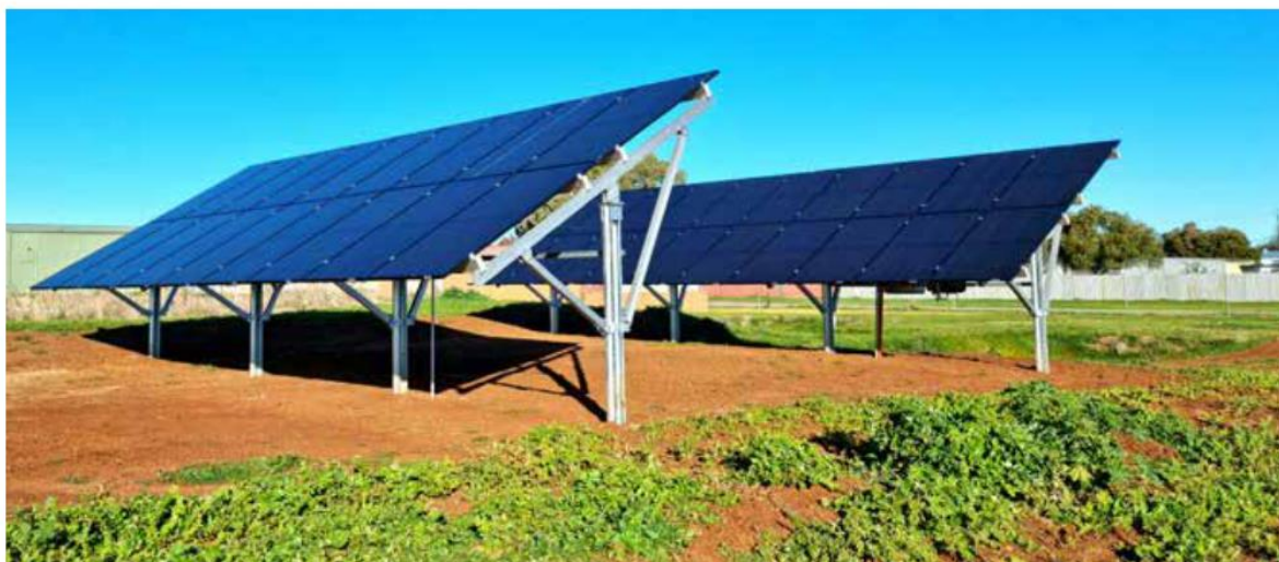
Whitton solar installation at Whitton Sewer Pump
