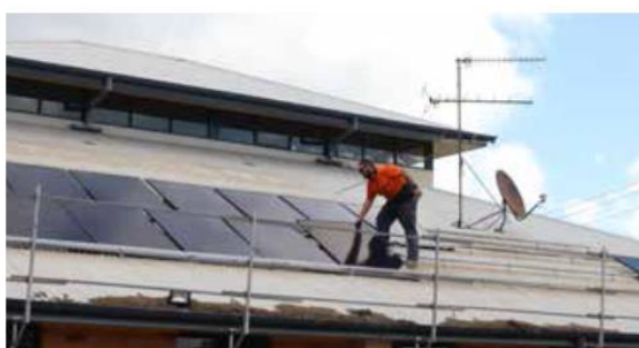
Solar panel installation at the Leeton Shire Library Installation completed by Ben Walsh Solar and Electrical
