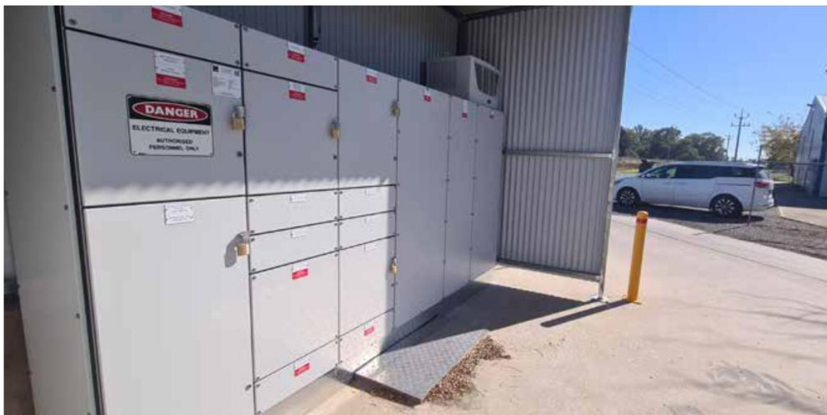
ClearScada System upgrade
