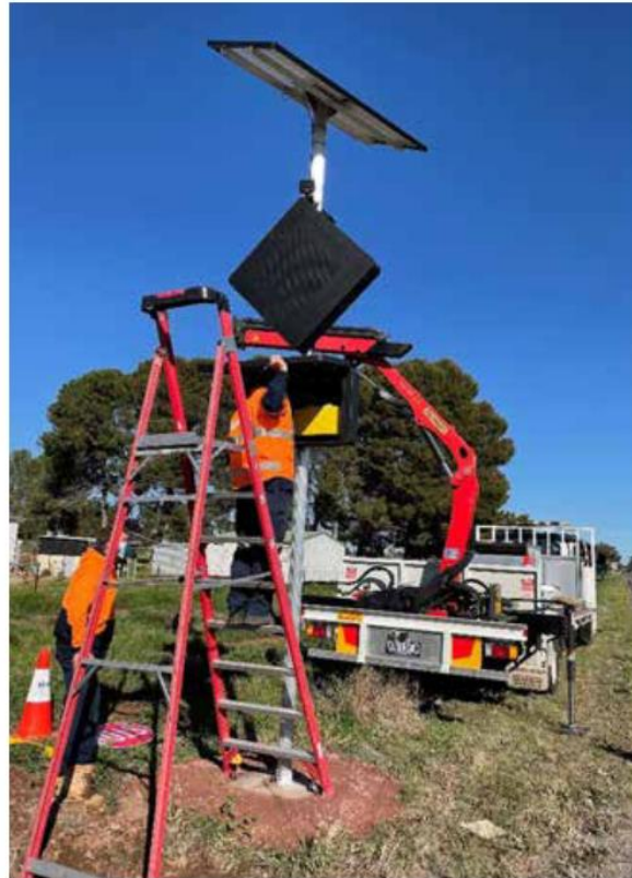
Vehicle Activated Signage installed on Research Road
